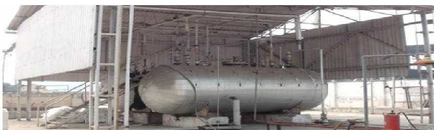
Figure 4. Ethylene Oxide Storage Tank (Capacity 10 tonne).
